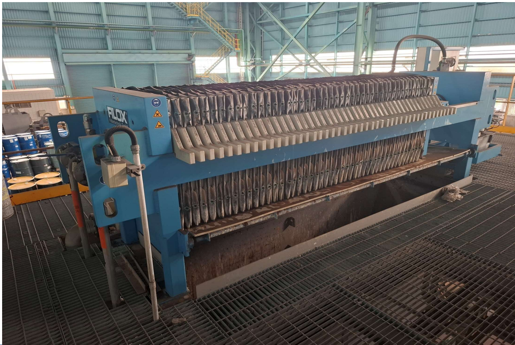
AT03-F02，材質鐵，4148.57KG，FILTER PRESS，二樓
